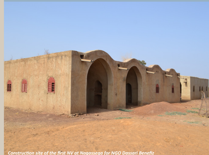
Construction site of the first NV at Nagassega for NGO Dassari Benefiz
