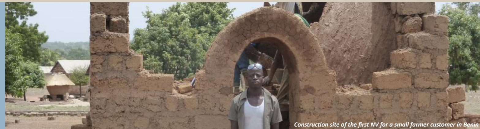
Construction site of the first NV for a small farmer customer in Benin
